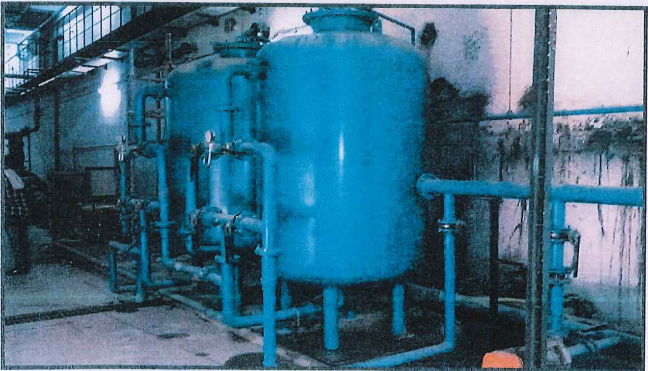
Multi Grade Filter & Activated Carbon Filter
