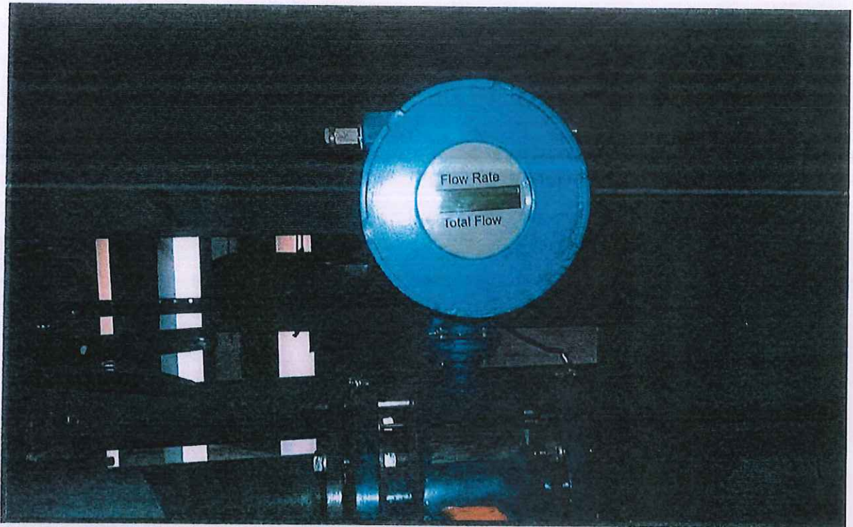
Inlet Flow meter
